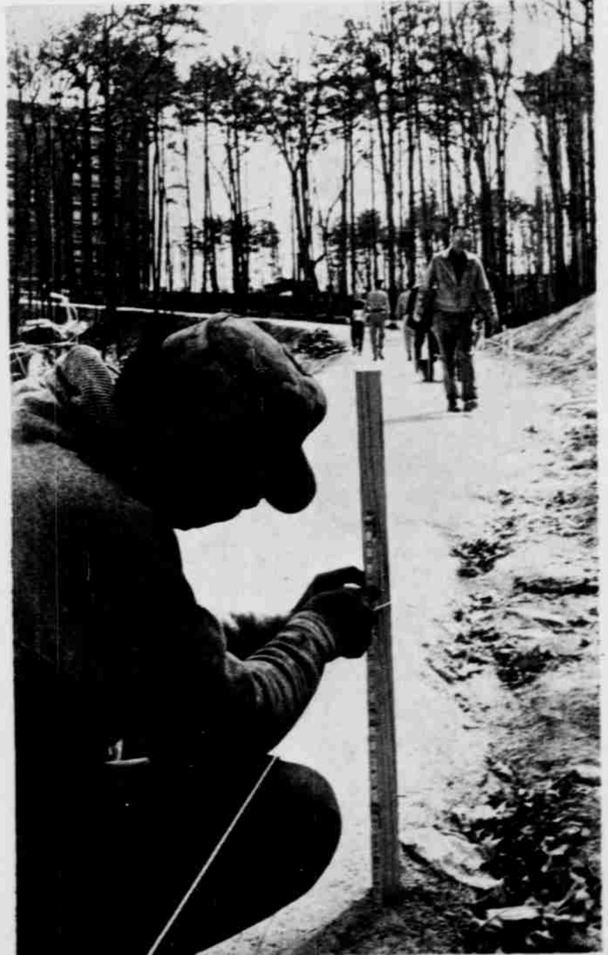
A SIDEWALK AT LAST! Work started yesterday on the sidewalk between Morrison and Kenan Fieldhouse. Here a worker is setting up a string to make sure the walk is straighter than the one Morrison residents built last week. Bricks in the background were part of the old walk which was taken up Tuesday.
