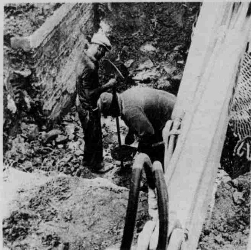
RIGHT NOW IT'S just a big hole next to the Bell Tower, but when completed it will house power and telephone lines. Tar Heel Staff Photo by Gene Wang
