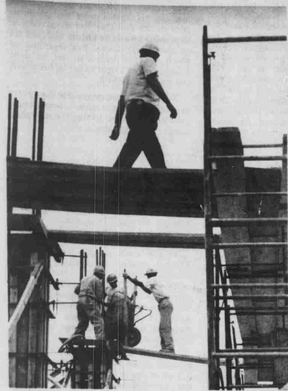
Workmen walk the scaffolds with wheel barrows full of cement as construction keeps rolling along on the Bingham Hall Annex. The fellow under the cement spout moved when the next wheelbarrow came up, but we don't know for sure.
