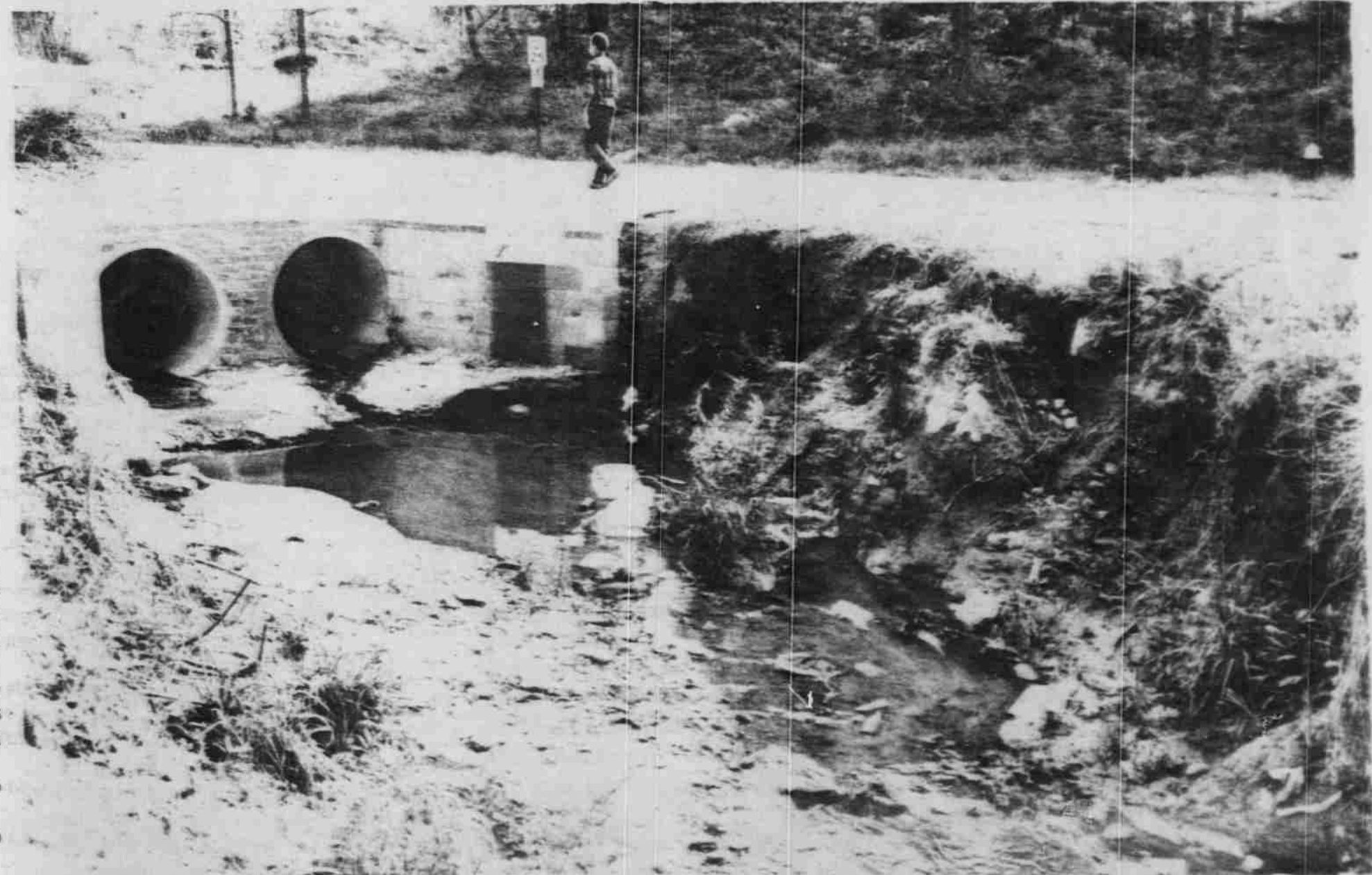
Passerby Crosses Drainage Ditch ... clogged by sewage from residences
