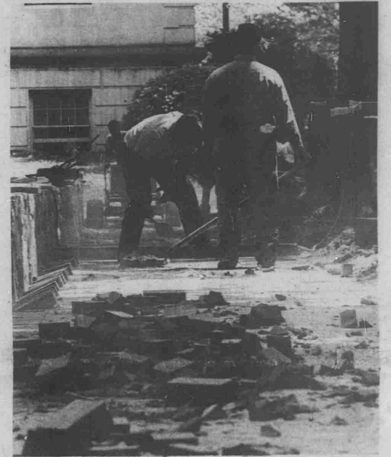
Polk Place will soon be a major thoroughfare for automobiles on campus from the looks of the work done recently by University workmen. These gentlemen were building the second of what appears to be a two-lane highway in front of Dey Hall Monday. (Staff photo by Leslie Todd)
