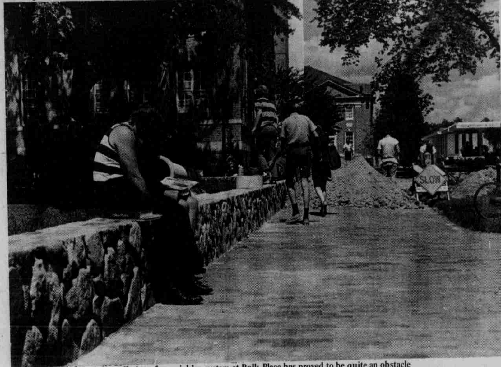
The installation of a sprinkler system at Polk Place has proved to be quite an obstacle course for pedestrians. So much, in fact, that the physical plant saw fit to put a traffic warning sign in front of the construction area. (Staff photo by John Gellman)
