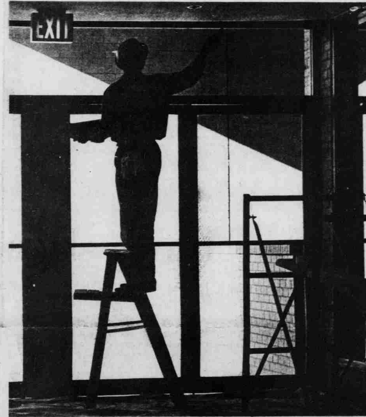
With a quick glance it looks like a little ballet on top of a ladder; but it is only part of many months of construction nearing the final stages as the new NCNB corridor opens up into a new shopping plaza. (Staff photo by Tad Stewart)
