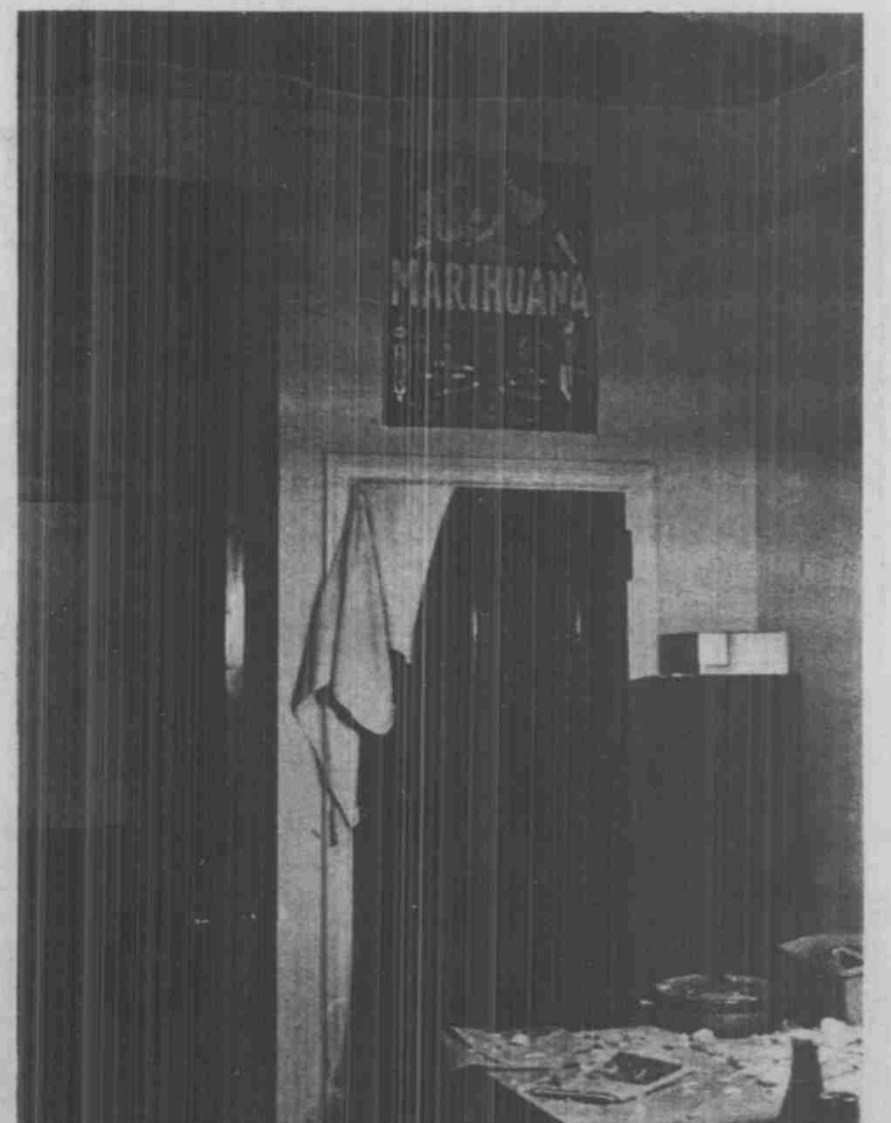
Residents of this quaint little room in Stacy dorm came home one day to find their ceiling had collapsed. After two weeks of hassling with the University, relief is still on the way. See story at left.
