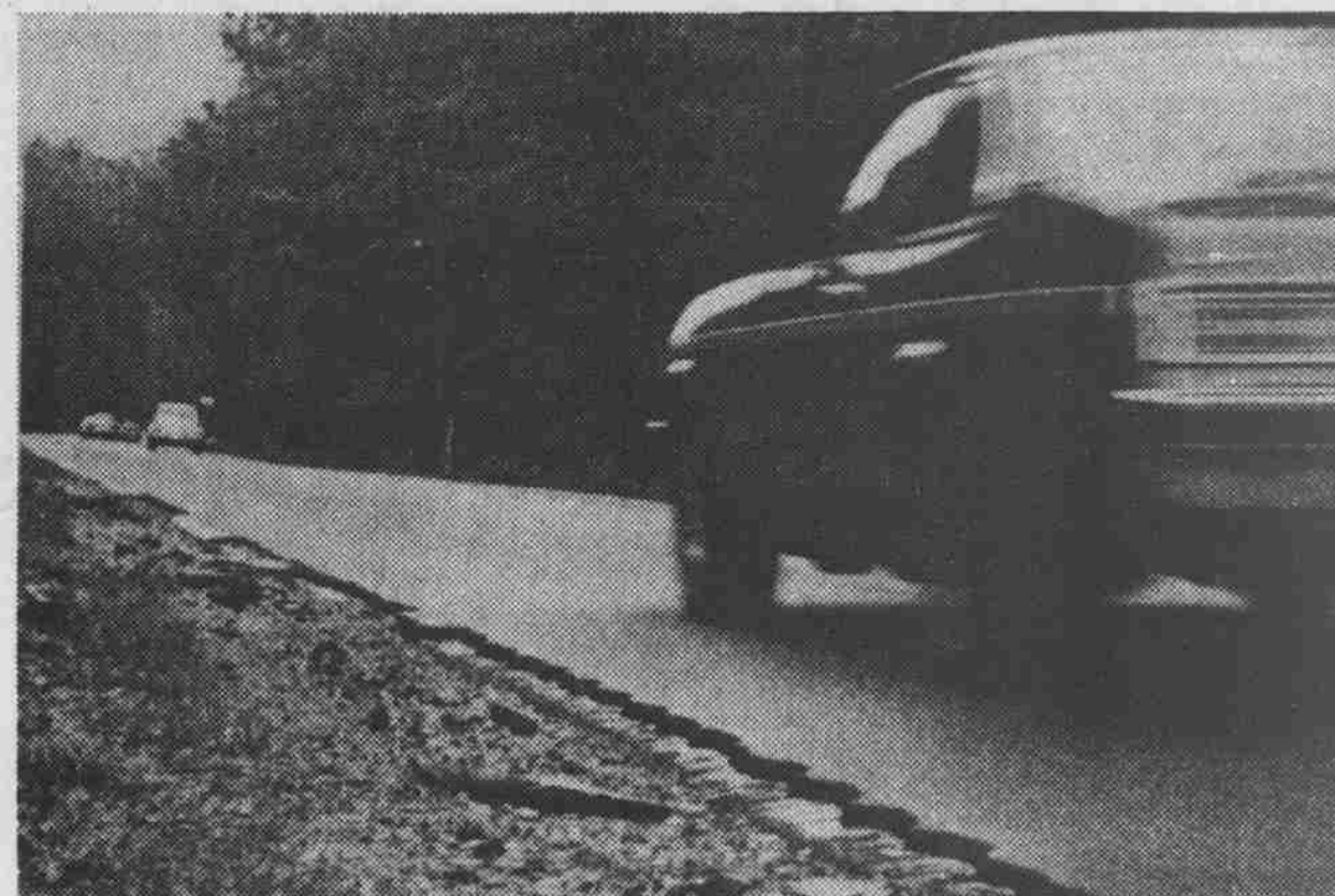
Rotten shoulders abound along N.C. 54 between Chapel Hill and Raleigh. Staff photo by Bruce Clarke
