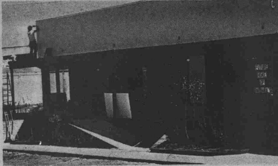
Builders work on expanding Kroger Plaza in Chapel Hill ... five businesses will move in by early 1982
