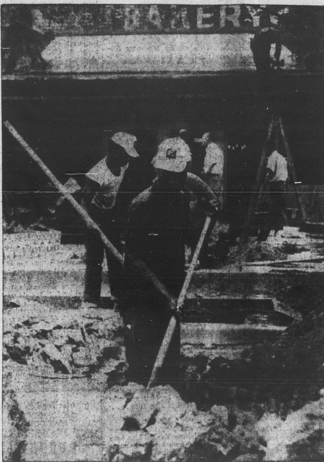
PUTTING UP A FRONT — Two businesses on Franklin Street are getting a new front. The businesses are Thell's Bakery and University Florist. The new front will be of Colonial design, with planters in front of the display windows. Exterior renovation also is being done at Wentworth & Sloan Jewelry Company and at Chapel Hill Laundry & Cleaners on Franklin.
