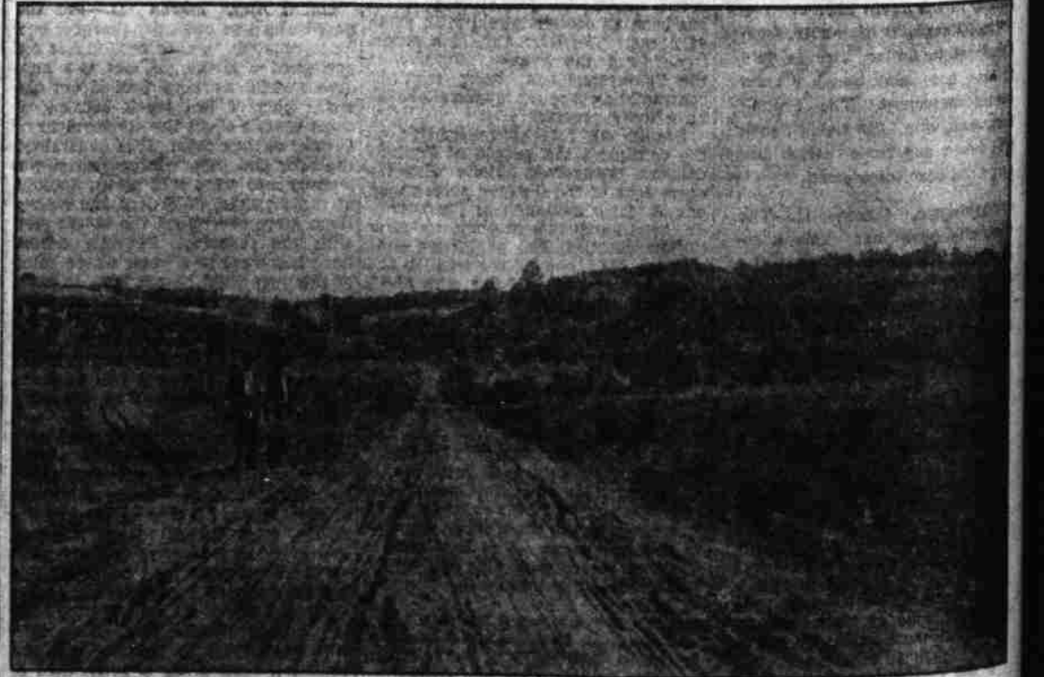
A stretch of highway on the Rural Hall road, near the Joe Marshall place, which is a good example of sections all over the county where the supervisor could use a road drag to good advantage.
