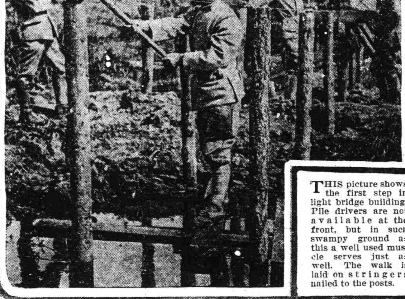
THIS picture shows the first step in light bridge building. Pile drivers are not available at the front, but in such swampy ground as this well used musclic serves just as well. The walk is laid on stringers nailed to the posts. (Pictorial Press Photo.)
