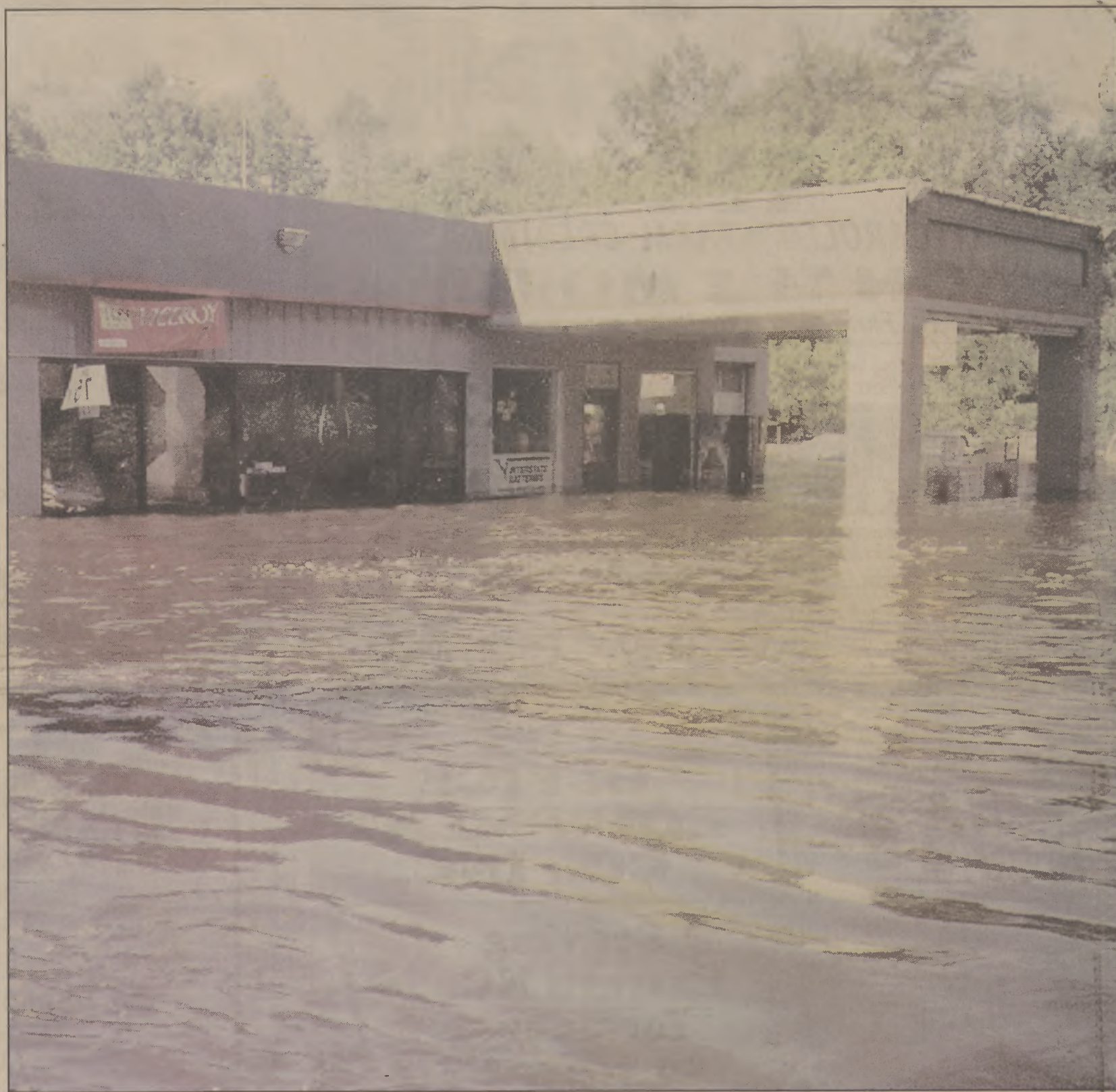
The water had begun to subside when the photo was made at Roy's Service Center, but the high water line can be seen on the side of the building. On the north side of town on U.S. 13 the Stocks' family home was also threatened, but damage there was minor compared to the loss of stock and equipment at the station. (Photo by Gina Rose)
