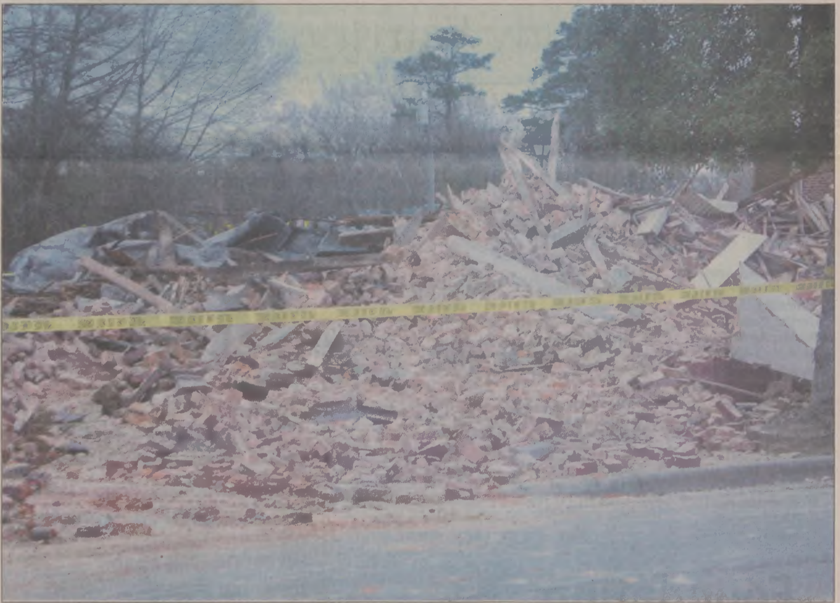
By early Sunday evening, all that was left of the former Western Auto building on Granville Street was a pile of rubble.
