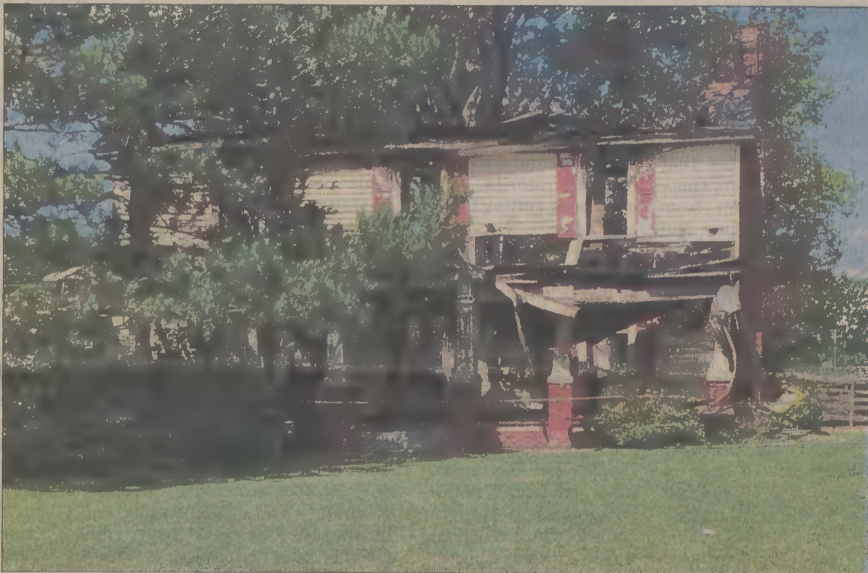
This house on Main Street in Roxobel was destroyed by fire the weekend of May 30. The home was a complete loss, but there was reportedly no injuries. The Roxobel Volunteer Fire Department was the lead agency for the fire.
