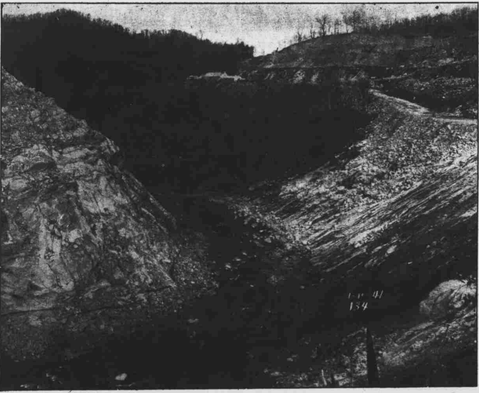
This shows both abutments of Nantahala Dam after they have been thoroughly cleaned, preparatory to actual construction of the dam. In the upper right of the picture can be seen the large power shovels and some of the shops of the Utah Construction Company.
