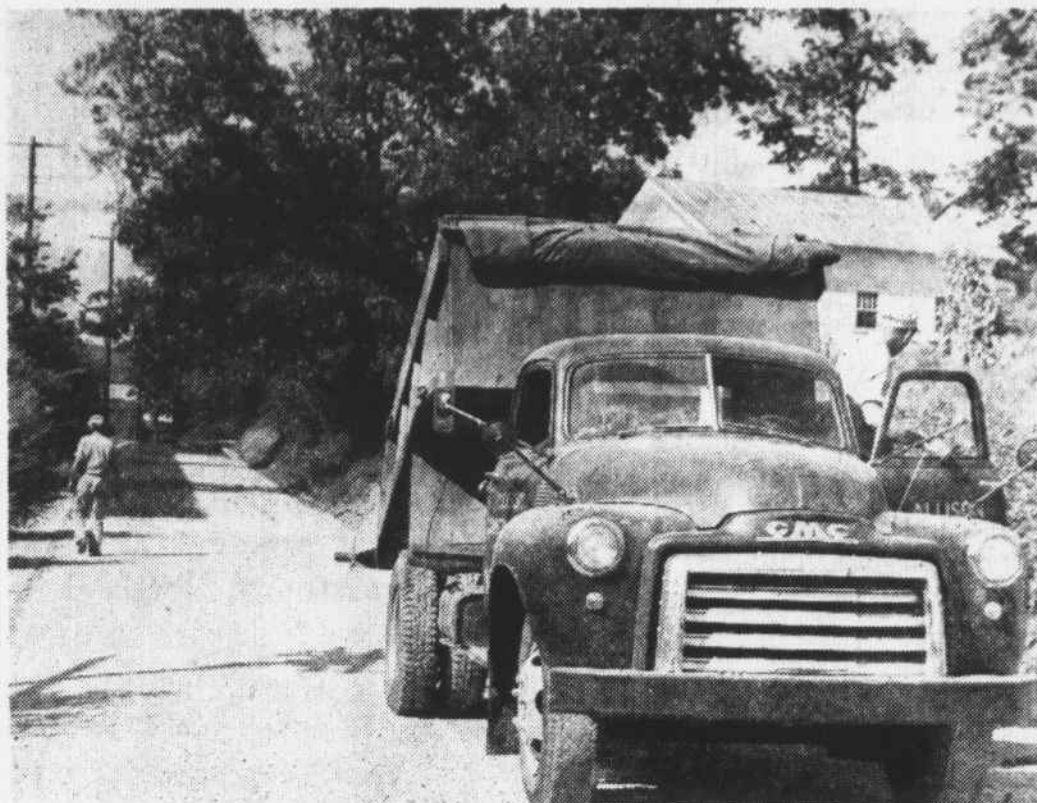
Workmen are shown putting the finishing touches on Green street, one of four Franklin streets surfaced this year with Powell Bill funds. The town is about a mile and a half short of reaching the half-way mark in having all its streets paved. The black section in the background is a portion of the street that had been tarred but not graveled. The four streets were surfaced at a cost of $12,422.43.
