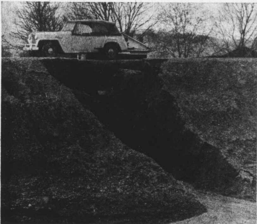
Recent rains washed out some shoulder sections along the new roadbed of the Franklin-Georgia link of US 23-441. Crews are now at work repairing the damage and preparations are under way for paving the 12.46-mile link. The pictured washout is near the Union cutoff.
