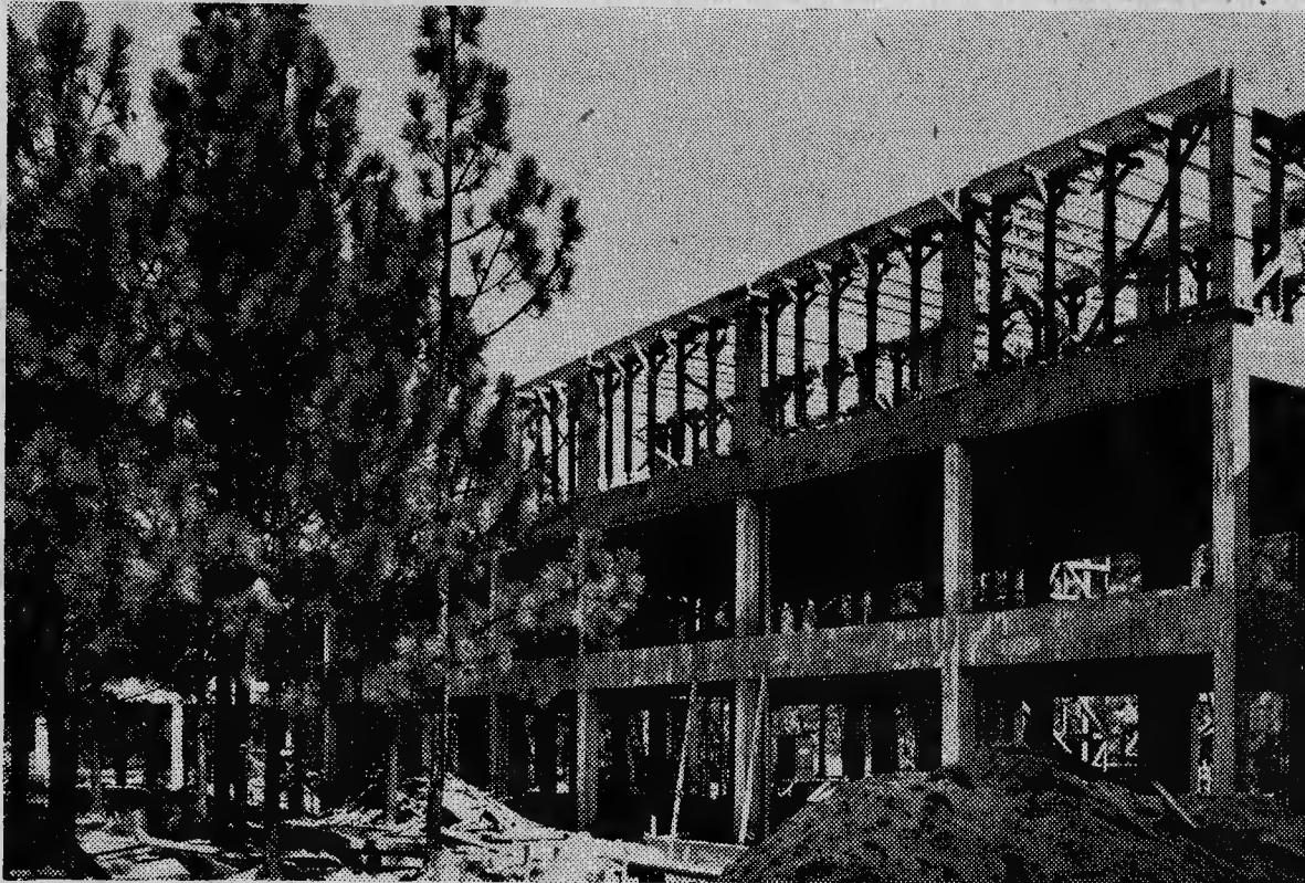
It's on the way, that new wing to the Moore County hospital which is slated to expand the hospital facilities far beyond what they are today. (Photo by Hemmer)
