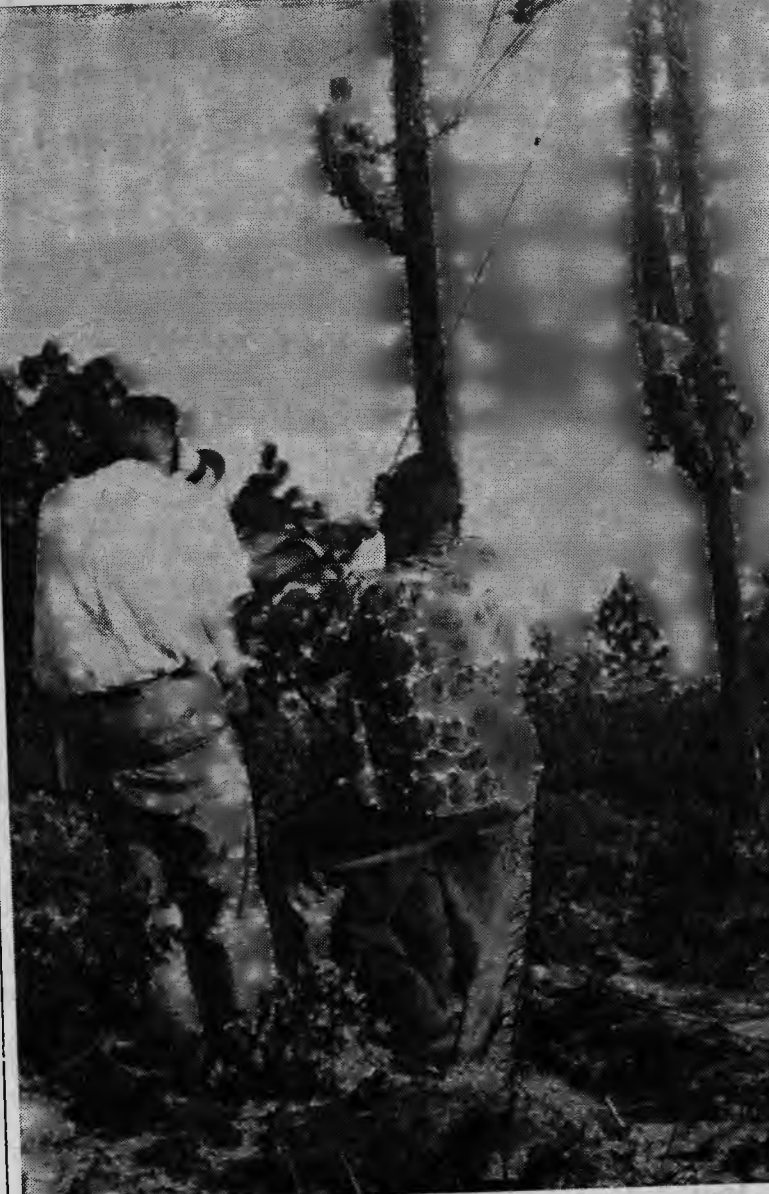
HOT WORK. Men on the ground pull hard to get the high-voltage line into place, in a temperature of well over 100 in the sun. Rear views shown above are those of Howard Fuquay and Page Choate. Just visible are the arms and gloved hands of Frank Leake Waddell, janitor at the Southern Pines division office who was impressed into service along with practically every other able-bodied employee of the CP&L. (Photo Geo. Sherrerd)
