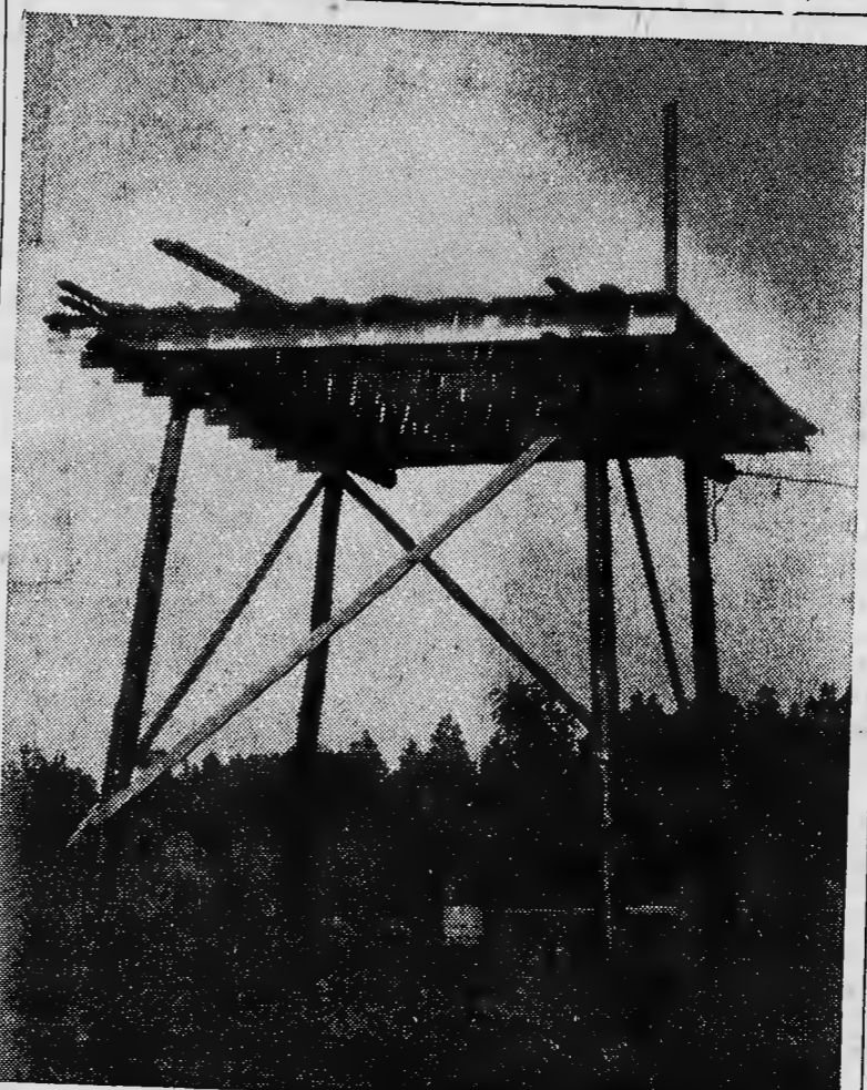
OBSERVATION TOWER for the Moore County Ground Observer Corps is still unfinished. The tower, located on the Boyd Estate, will play a vital part in "Operation Skywatch" for eastern defense of the country in the event of an enemy attack, according to Dave Drexel, county supervisor of the GOC. Volunteers who would like to help complete the construction should contact Fred Hall, Jr., chief construction engineer, Harry Chatfield, chief observer, or Col. George Garde, post supervisor. When completed the tower will have a closed-in room and adequate facilities for complete hookup with Ground Observer Corps posts in other sections of the area. (Pilot photo)
