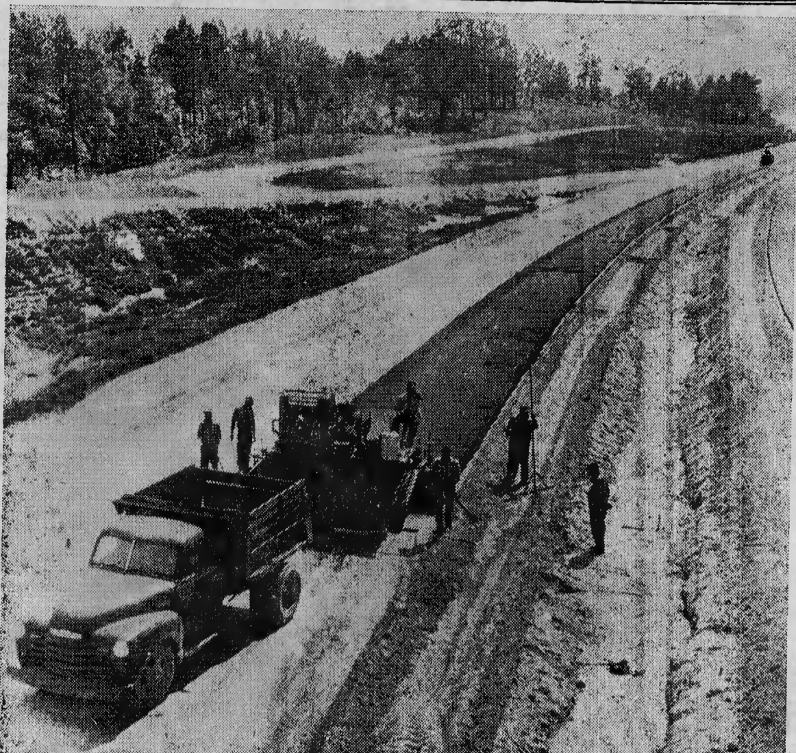
THRUWAY PAVING continued this week, a bit behind schedule, as workmen started moving to the south end of the project. Pictured here is the machine that lays the hot asphalt. The truck dumps its load into the hopper of the paver, then remains as the asphalt is distributed in smooth layers over the sand-clay base. The picture was made from the Pennsylvania Avenue bridge. (Pilot photo)
