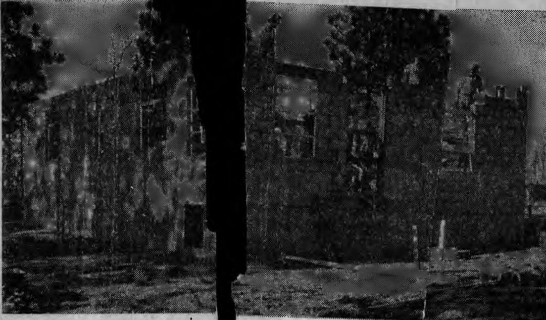
GOING UP—The new home built by friends, neighbors and other volunteer workers for the Robert Kennedy fund was started Monday only a few days after work was started. The roof was put on today. Arl Danly, chairman of the building committee for the South Pines Moose Lodge, who is supervising construction, can be seen in upper right corner of picture. (Humphrey photo)
