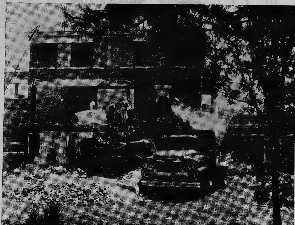
HOSPITAL WORK STARTS — This was the scene at Moore Memorial Hospital as workers of the C. P. Street Construction Co. of Charlotte, prime contractor, were tearing down the former medical records room at the point where the big new surgical wing of the hospital will join the west end of the existing building. (Hemmer photo)
