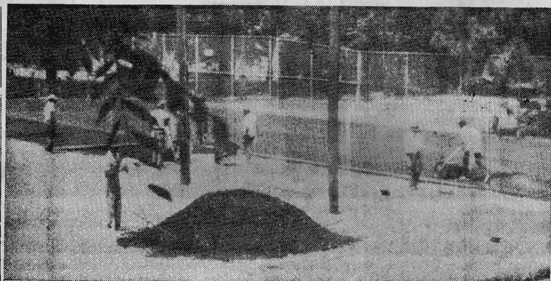
NO MORE MUD! —A black asphalt base is being rolled onto the town courts, on which a green composition surface will be applied, making tennis an all-weather, all-year-round sport here. One court was completed last summer and the other three are being surfaced now. (V. Nicholson photo)
