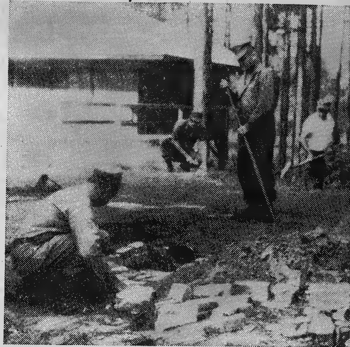
BRICK-LINED CULVERTS are completed on both sides of cabin road, with drainage ditch dug down hill on far side.
