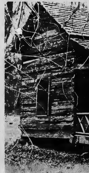
OLDEST STRUCTURE? — This cabin, the kitchen of James McLendon, built in 1760, is one of the oldest, if not THE oldest, structures in Moore County. The late Rassie Wicker identified the cabin, near Harris Crossroads on the Pinehurst-Robbins Road as possibly the oldest in Moore County. It was given to the Moore County Historical Society along with the nearby home of James Bryant several years ago. Harris Blake, a director, was chairman of an ad hoc committee which has obtained old boards to repair the Bryant House, repaired a sagging chimney, and boarded it up for protection. One of Mr. Wicker's dreams was restoring what he called a "fine example in an almost perfect state of preservation" after 200 years. McLendon's mill stood nearby, and was an early settlement of Scotsmen. (Photo by Glenn M. Sides).
