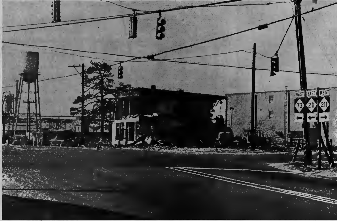
DESTRUCTION FOR PROGRESS —This block in the center of West End was demolished last week to make way for the addition of a two and a-half million dollar expansion of the Sandhills Division of the Stanley Furniture Co., a Mead concern. The ground breaking is Thursday.
