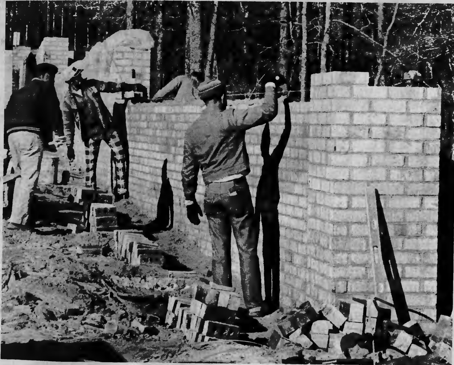
CONDOMINIUM SITE CONSTRUCTION — Workmen are shown putting the finishing touches on a three-third mile long wall which will enclose a new multi-million dollar condominium project now under way on Morganton Road opposite the Country Club of North Carolina. —(Photo by Glenn M. Sides).
