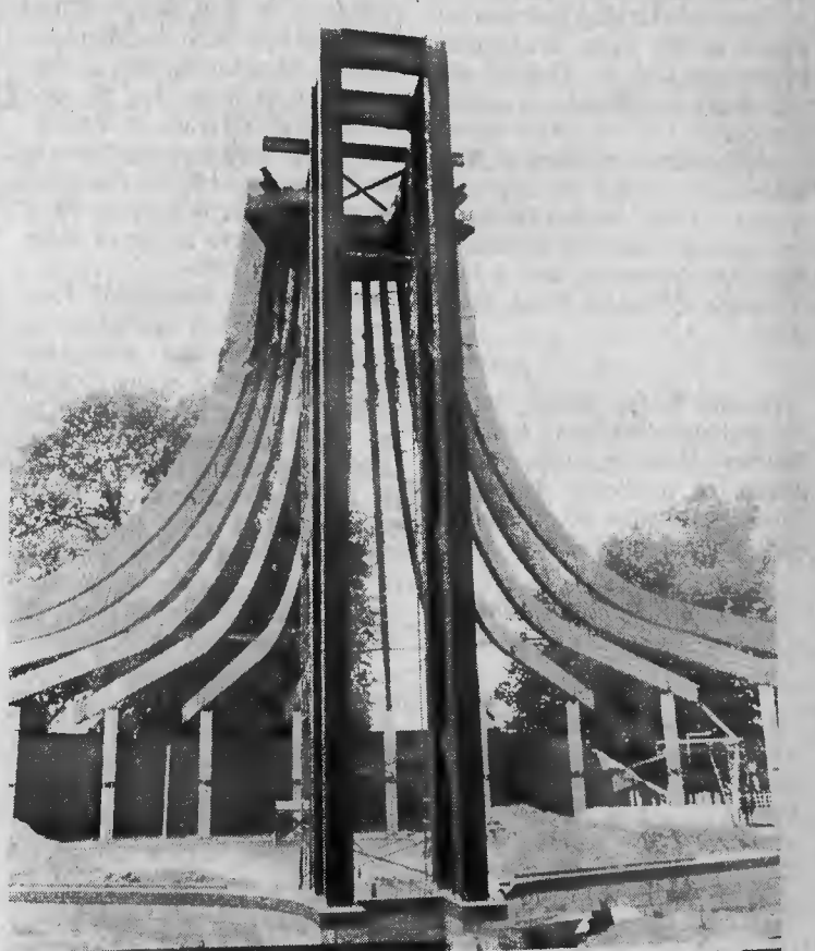
CHURCH UNDER WAY — This striking photograph by Glenn M. Sides shows the St. Anthony's Catholic Church under construction here. The unique design of the church will be constructed so that all worshippers will be equi-distant from the altar.
