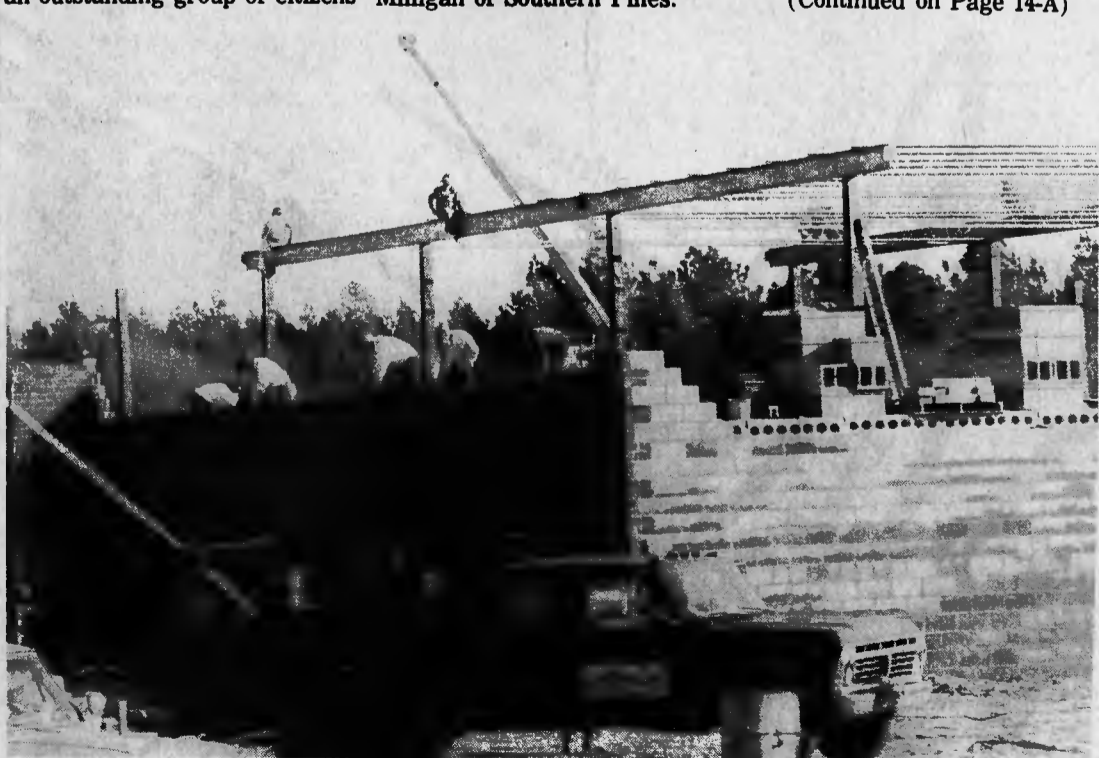
OPENING IN MAY — Construction is well under way on the new HOW plant at the old airport Industrial Park near Aberdeen, with the textile manufacturing firm scheduled to start operations in May. A German-owned syndicate, HOW's operations here are headed by Bernhard Schuler.—(Photo by Glenn M. Sides).
