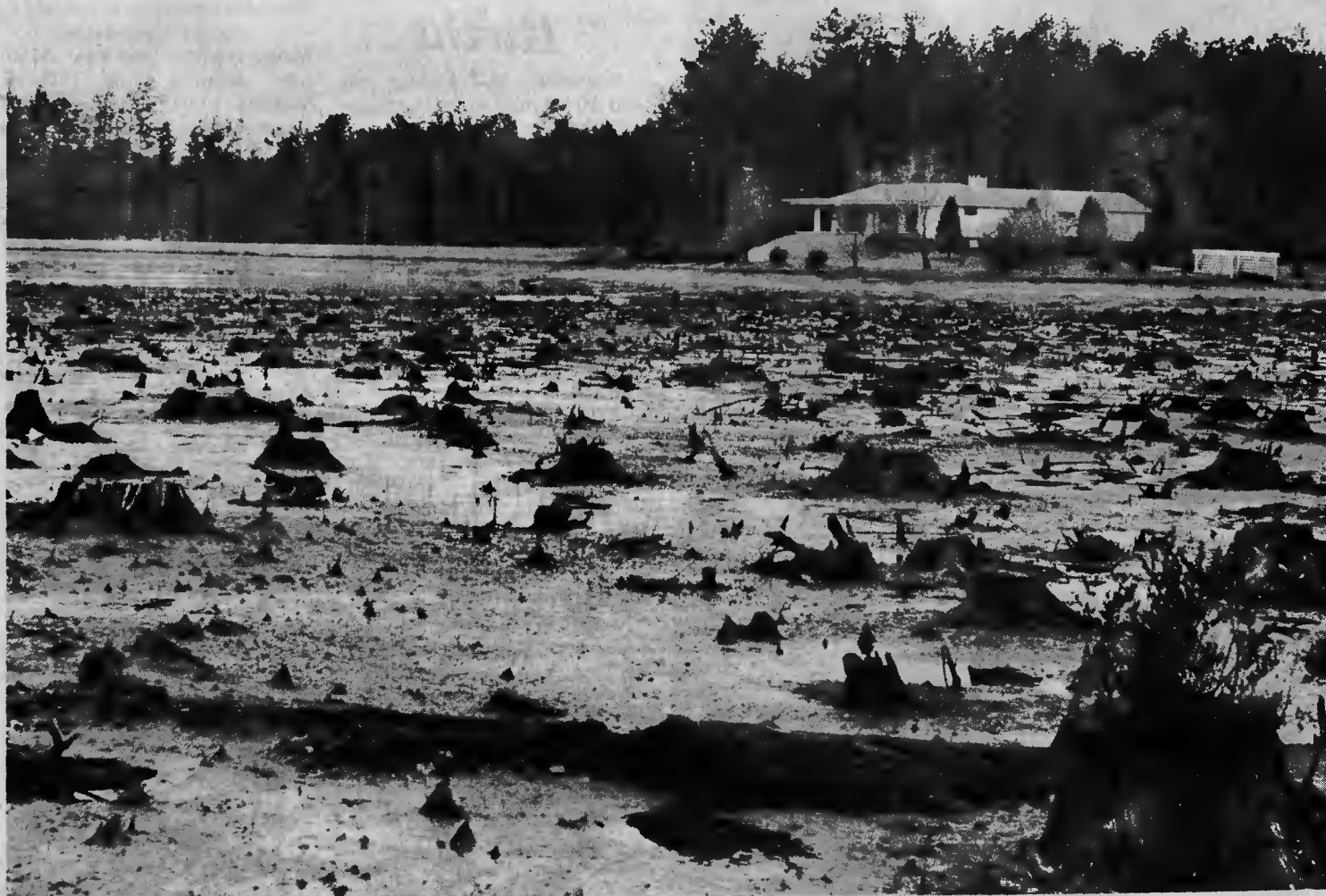
DRAINED LAKE — This is one of the two lakes at the Country Club of North Carolina that were drained to aid in construction of the regional sewer system. This lake beside US 15-501 will be refilled later this month but the other will remain dry until the completion of the project in April.—(Photo by Glenn M. Sides)
