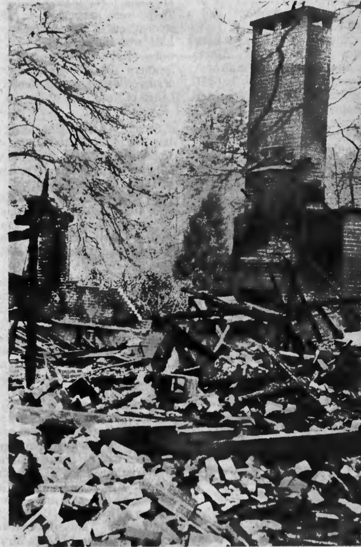
ARSON CHARGED — This is what remains of the Edgar B. Smith home at 605 Midland Road following a second fire, in which Robert L. Stuart Jr., 18, is charged with arson.—(Photo by Glenn M. Sides).
