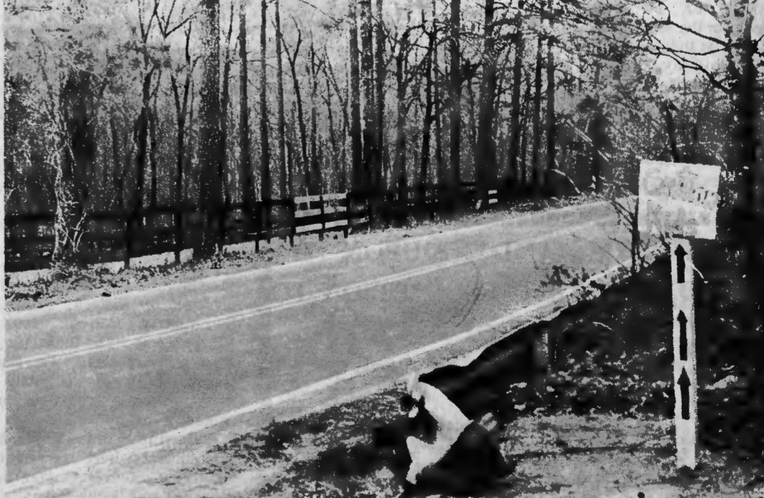
FENCE A TARGET — This fence along the property of Dr. and Mrs. Anthony G. Hucks-Folliss on East Connecticut Avenue has been a special target for automobiles failing to make the curve at DunCraig Manor, where the sign at right was erected. Mrs. Hucks-Folliss said their fence has been knocked down five times in the past three months, the latest this past Friday night.
