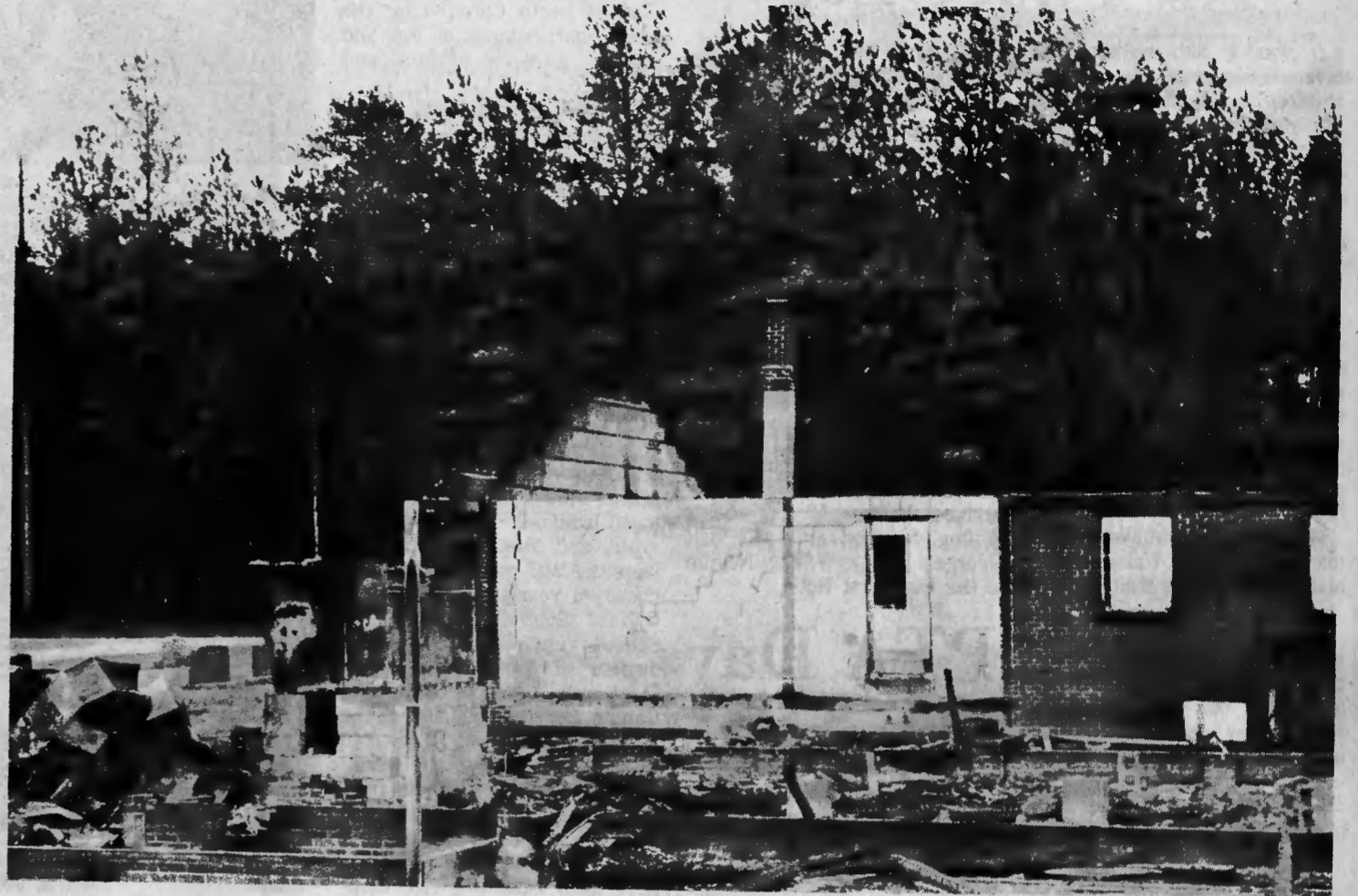
FIRE DESTROYS CHURCH - This is all that was left this week of Bethlehem Church, the oldest Baptist Church in Moore County, after fire swept the sanctuary and educational building early Sunday morning. The only thing left was part of the walls of the educational building. - (Photo by Michael Valen)
