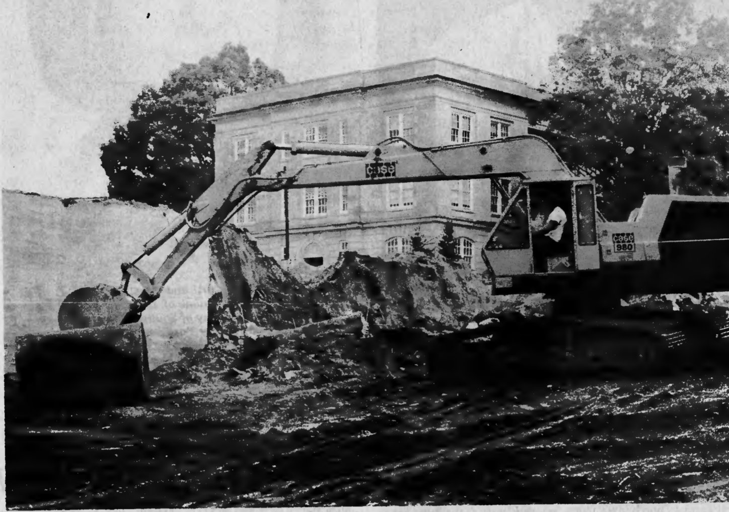
COURT FACILITY SITE — Work got under way this past week on clearing the site in preparation for the beginning of construction on the new Moore County court facility. The present courthouse is in the background. Completion date for the new court building is after 510 work days. — (Photo by Glenn M. Sides).
