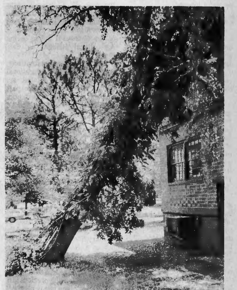
STORM RESULT — A sudden thunderstorm with strong winds hit Southern Pines late Monday afternoon and uprooted some trees, including this large one which fell on the building housing the architectural firm of Austin Associates on E. Connecticut Ave.
