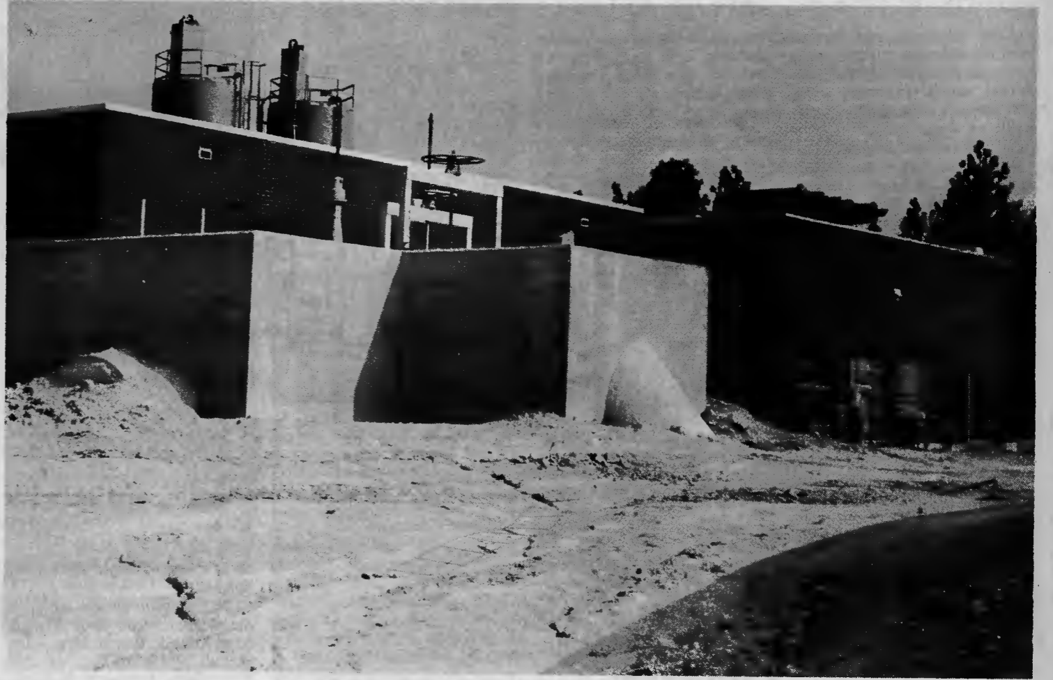
IN OPERATION DEC. 1 — This is one view of the giant processing plant near Ador for the Moore County regional sewer system which is scheduled to go into operation on Dec. 1. The waste disposal treatment plant will serve Southern Pines, Pinehurst and Aberdeen. —(Photo by Glenn M. Sides)
