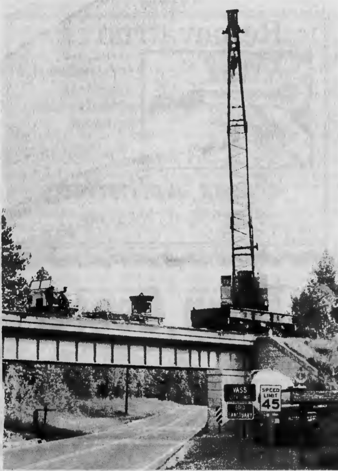
BRIDGE WORK — An unusual operation has been taking place at this railroad overpass on U.S. 1 at Vass this past week. A new trestle is being built across Little River by the Seaboard-Coast Line and to get the concrete to the trestle site required a huge crane which dropped a big bucket to a truck, shown at left, and then transferred it to a railroad car.—(Photo by Glenn M. Sides).
