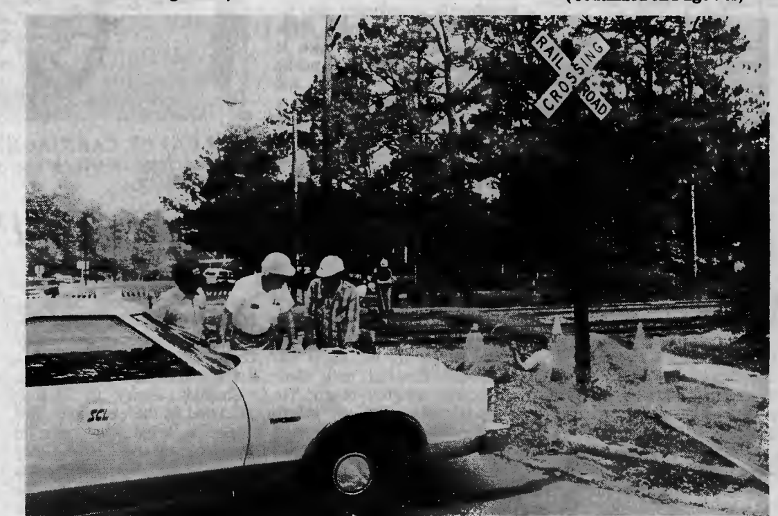
CROSSING SAFETY — The long delayed work of making the dangerous New York Avenue railroad crossing safer got under way in Southern Pines this (Wednesday) morning. It is expected to be completed in a couple of weeks. The project was expedited through the efforts of Congressman Bill Hefner.—(Photo by Glenn M. Sides).
