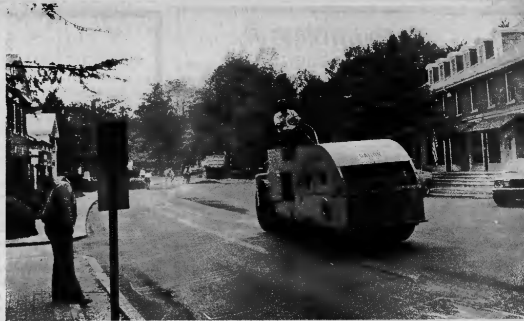
RESURFACED — The two main streets of Pinehurst were resurfaced early last week in work authorized by the Pinehurst Village Council. The flow of traffic through the town continued unabated, with the assistance of the local Police Department.—(Photo by M.E. de Nisoff).
