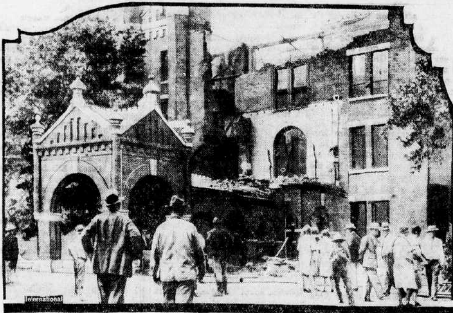
Administration building of the Central Hospital for the Insane at Nashville, Tenn., after the fire that swept through the institution. More than a thousand inmates were released to save them from the flames and thirteen were missing.
