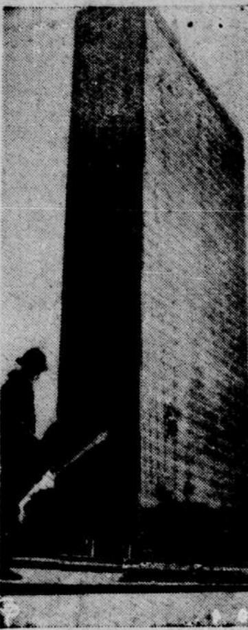
A UNITED NATIONS blueprint for building is studied by rivet foreman Joseph Jones as he balances on a girder of the new General Assembly and Security Council structure in New York. The completed U.N. secretariat office on East River site looms behind him. (International)
