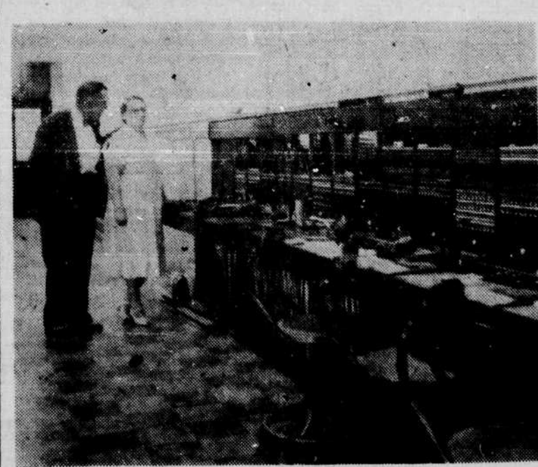
J. F. Havens of Tarboro, Vice President, and Mrs. Lucy Mobley of Williamston, Chief Operator, are shown above inspecting 4 additional operator's long distance switchboard positions being installed for service here by the Carolina Telephone and Telegraph Company. The new switchboard positions, boosting the number to twelve, were placed in service recently, increasing operating facilities in Williamston by 80 per cent.
