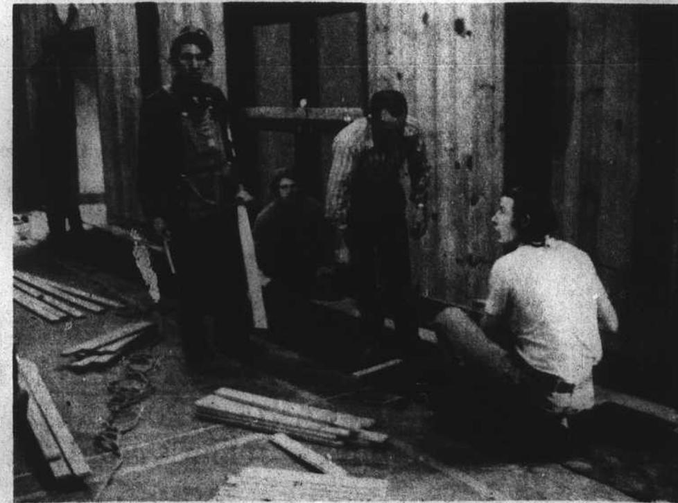
VOLUNTEER WORKERS PITCHED IN to install a hardwood floor in the Cashiers Community Center Recreational Hall. The above photos show Brad Pell, Duane Dillard, Ray Piantanida, Wayne Dillard, Johnny Hooper, Blaine Hawkins and Rex Allen.
