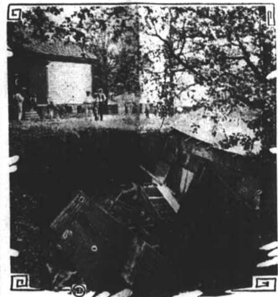
A number of mysterious cave-ins of land in Birmingham, Ala., have got the citizens all on edge. Here is a picture of one, where the ground opened and set a double garage, a coal shed and a large tree sink down into a hole. Scientists believe there are subterranean cavities under the city, and say the drainage of water from these cavities causes the settling.
