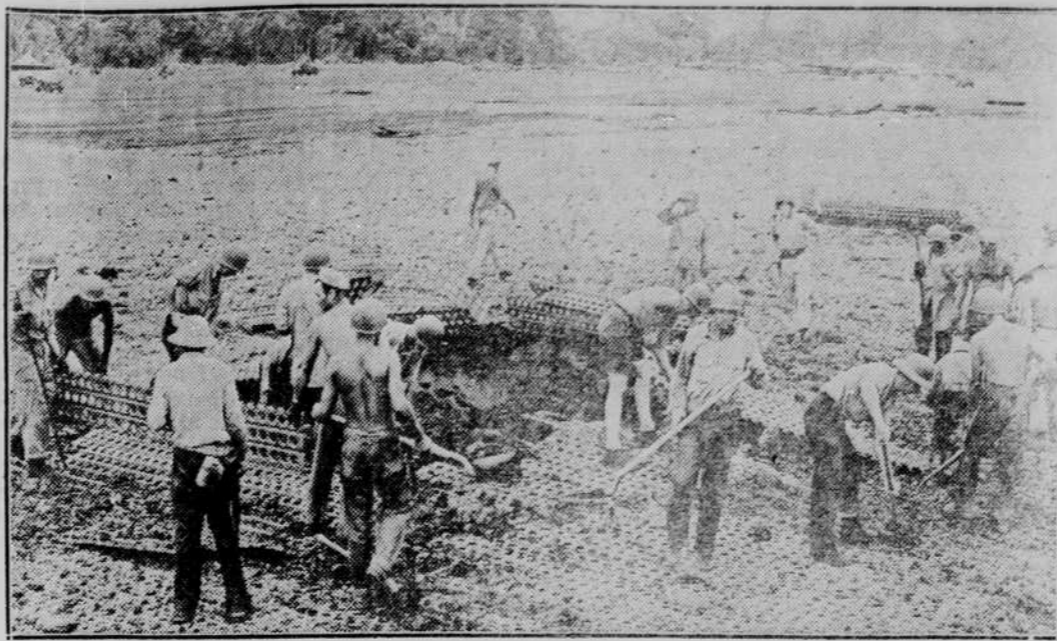
LIGHTNING REPAIRS OF BOMB DAMAGE —Sometimes it is merely a matter of minutes after enemy aircraft bomb an airfield until U. S. Army Aviation Engineers are on the job repairing the damage. The portable steel landing mat is replaced and the runways are available for American planes in the shortest possible time. This scene at Guadalcanal is typical of the efficient work in restoring a shattered airfield. The Seabees, naval counterpart of the Aviation Engineers, have made splendid records in this theater of operations.
