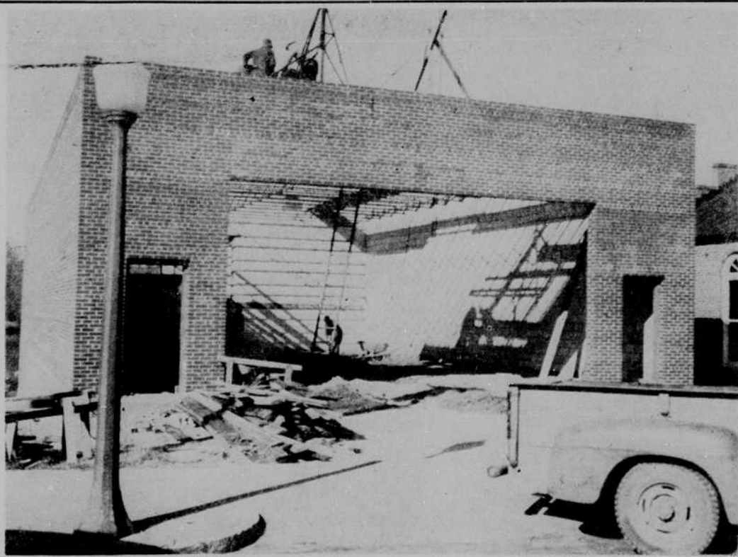
Plymouth volunteer firemen didn't get into their new home by the first of the year, as they hoped, but work is going forward and at least it won't be as long as it has been. The new building will have room for three pieces of equipment at the front, with a club room, showers, lockers and a work room for the firemen at the back. It is 40 by 90 feet overall and is built of concrete blocks with a brick veneer. Robert L. Tetterton is contractor for labor on the building, with the town furnishing all materials. Jack Liverman is the supervising architect.—Polaroid 1-Minute staff photo.
