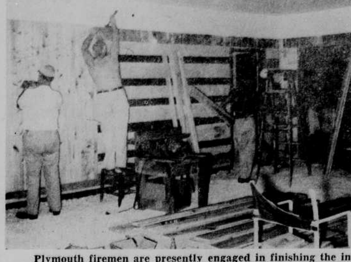
Plymouth firemen are presently engaged in finishing the interior of the new fire department building completed here some time ago. Several of them were installing the cypress paneling in the main clubroom when this photo was made last Thursday. That's Bud Lovic at the left doing some wiring, while Tom Sanderson, Harry Gurkin and Lawrence Jones (back of the ladder) are working on the walls.—Polaroid 1-Minute staff photo.
