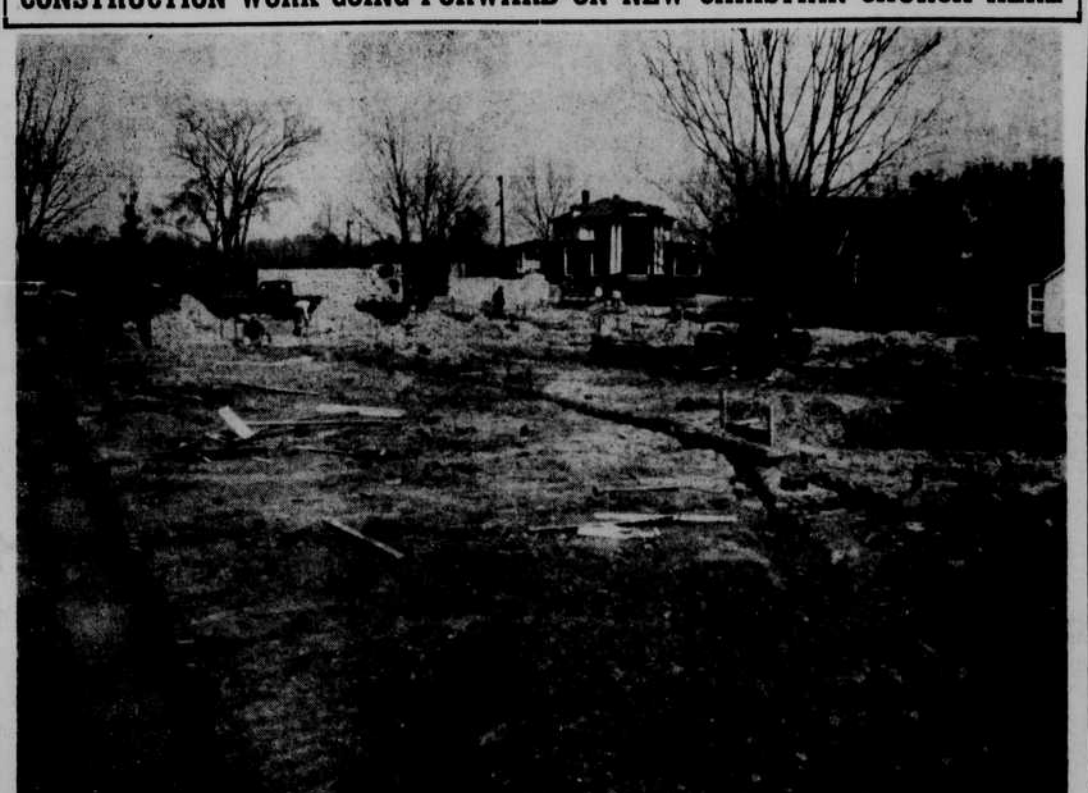
Work is progressing fairly rapidly on the new building for the First Christian Church of Plymouth. Practically all of the reinforced concrete foundations had been poured and masons were starting to place the concrete blocks last Friday, when the above photo was made. Located in the 300 block of East Main Street, the new church structure will extend practically all the way through the block to Third Street. Robert L. Tetterton is contractor for the building, which is to be completed and ready for occupancy by the end of February next year.—Polaroid 1-Minute staff photo.
